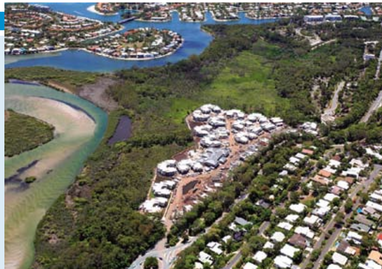
WORK is progressing well at Noosa Sanctuary with all of the 37 buildings under construction. The project is on time despite having two months and 2.6m of rain since commencement. The display unit is now open with a high level of interest in the end product. The Resort will be managed by Mirvac as Quay West Noosa.
